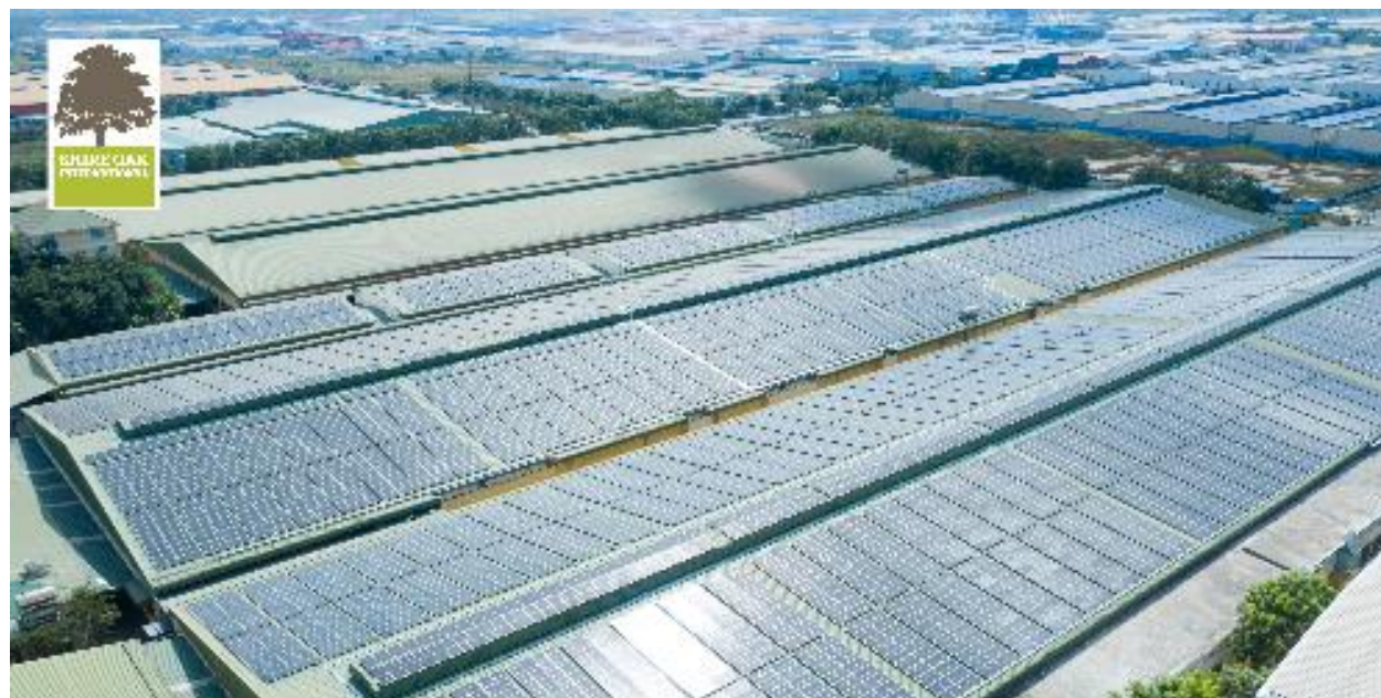
Dong Khanh, Long An | 4,977 kWp
