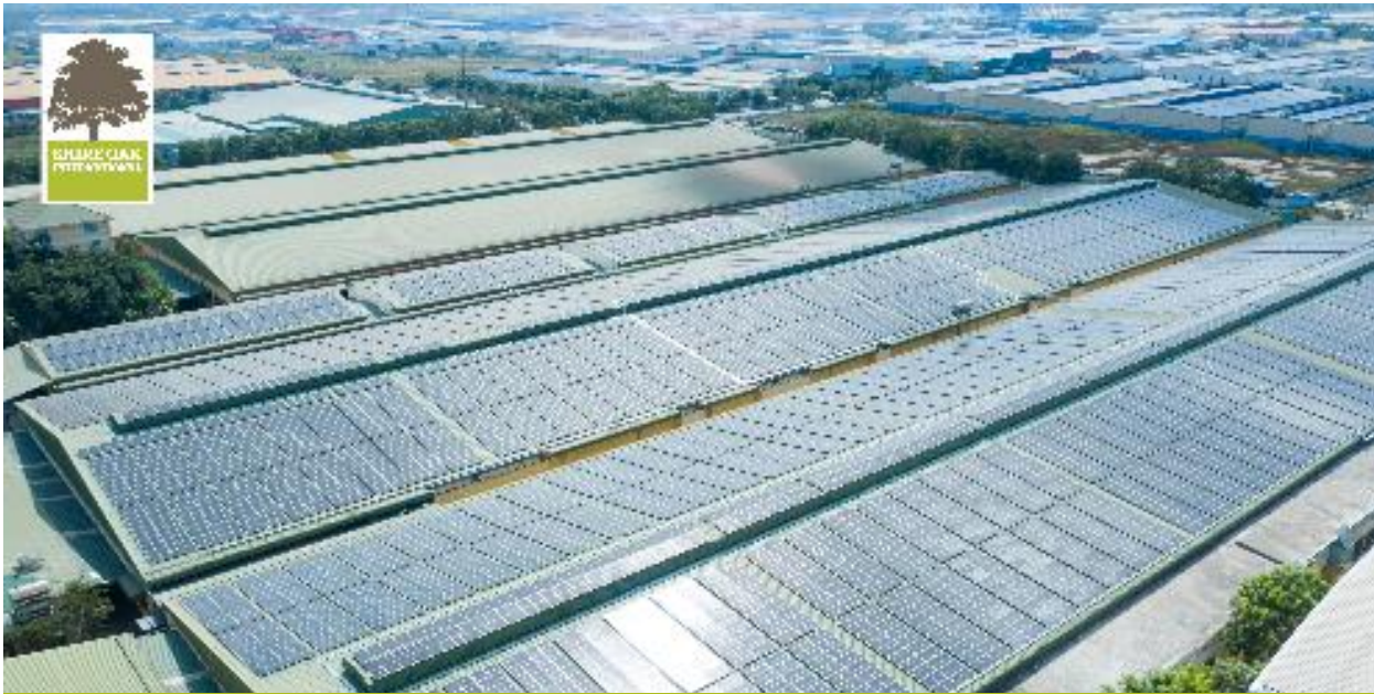
Dong Khanh, Long An | 4,977 kWp
