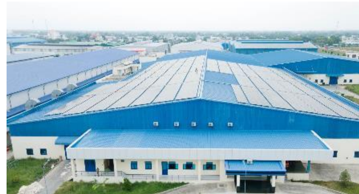
Viet Phu, Long An | 999.68 kWp
