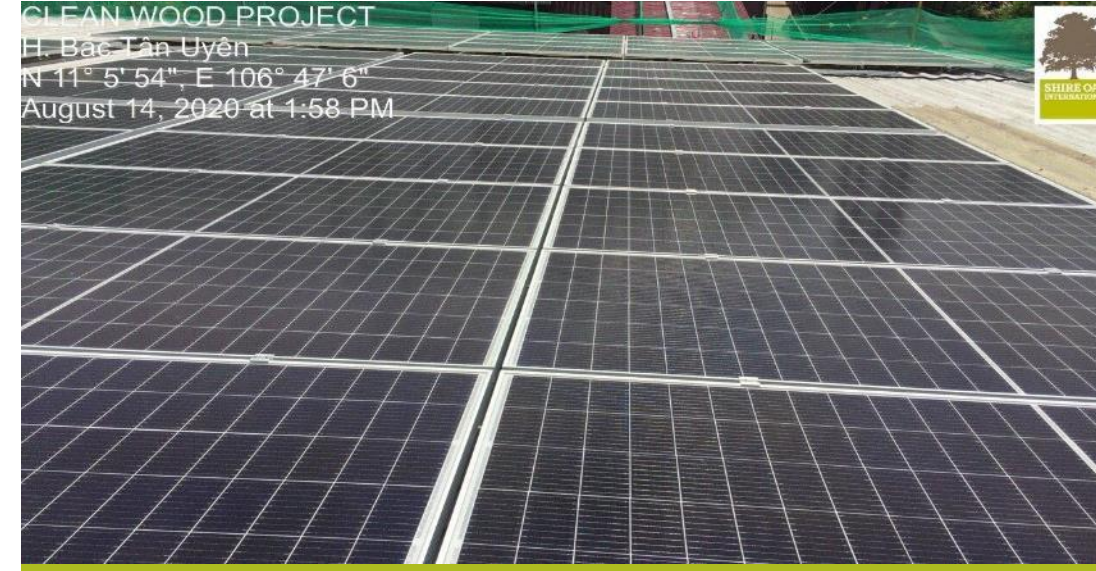
Clean wood | 760.32 kWp
